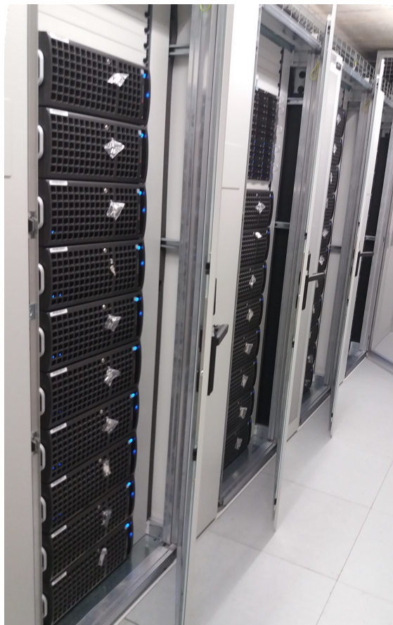
Figure 3.2: Server racks of the TCML-Cluster.
