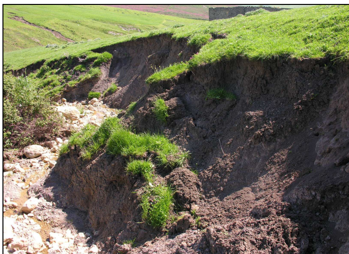
Figure 5.17. Bank erosion causing river walls collapse (12.05.2011).
