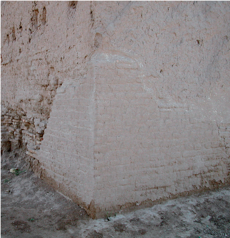
Fig. 6. Reconstructed corner of the Kepter Khana in the Shahriyar Ark of Sultan Kala, where new degradation through water absorption is becoming apparent at the base of the monument.
