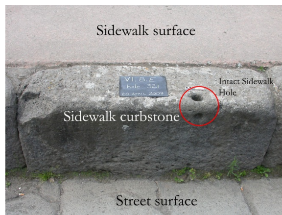
Figure 2. An intact sidewalk hole on the upper street-facing edge of the curbstone.
